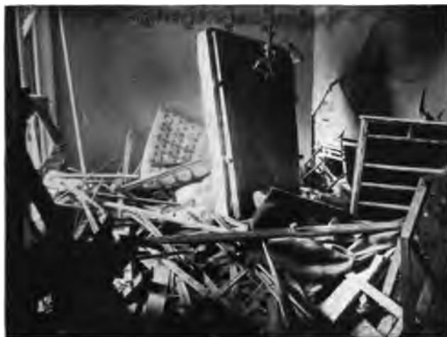
Fig. 3. Explosion of Low-Pressure Heating Boiler.
